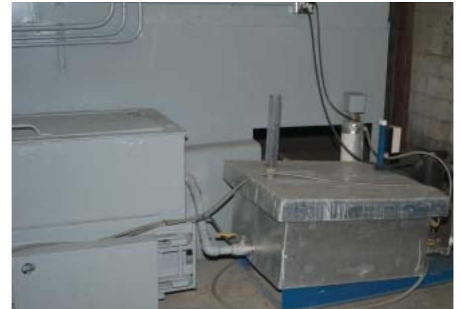
Metcam's new ultrafiltration membrane system installed on Metcam's five-stage pretreatment line continuously removes oil and grease from Stage 1, and ultimately reduces wastewater at Stages 1 and 2. Adding this system and a rinse crossflow system that ties Stages 1 and Stage 2 together reduces wastewater production by more than 76,000 gal./yr. and yields net cost savings for wastewater processing of more than $29,000/yr.
